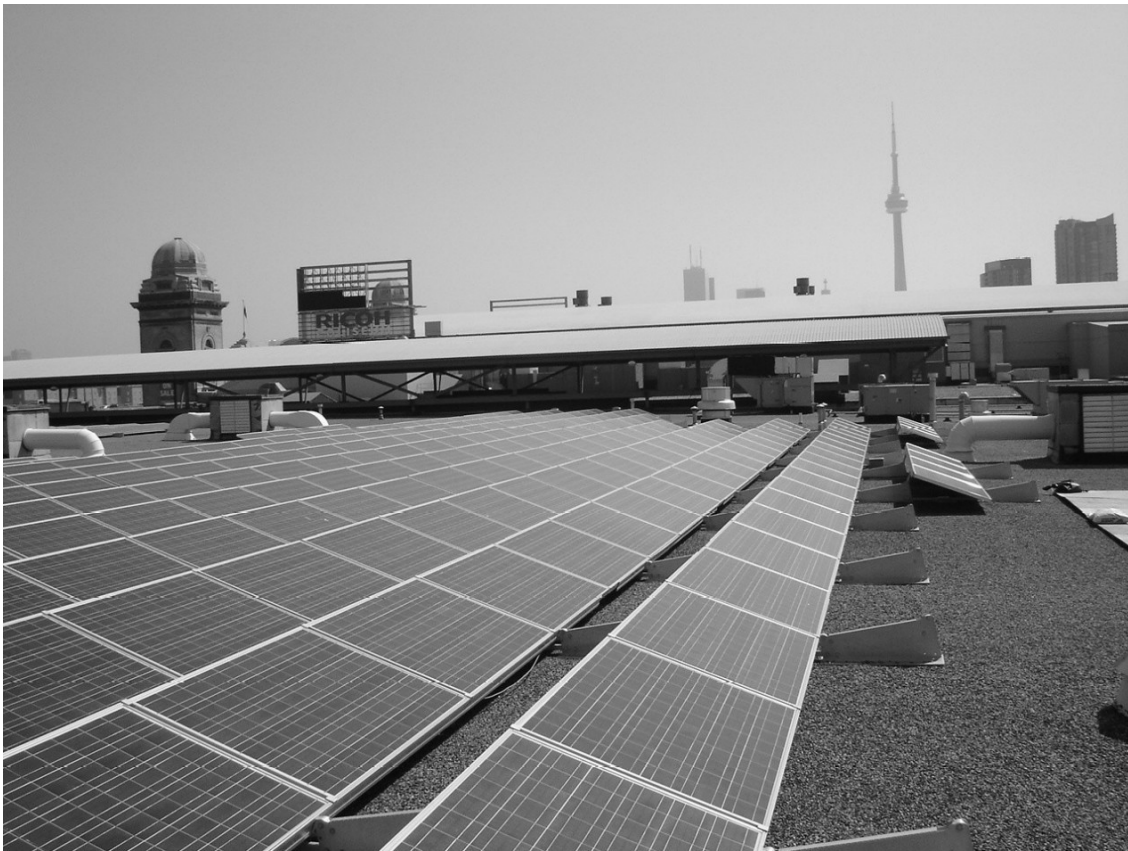
Figure 8: Solar roof at Exhibition Place
