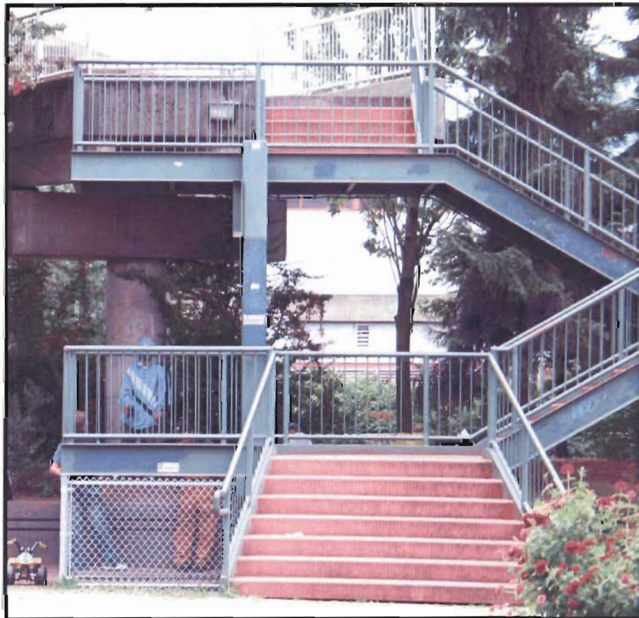
Pedestrian overpass connects Hyack Square with waterfront but is not usable by people of all physical abilities (Photo: J. Natland)
