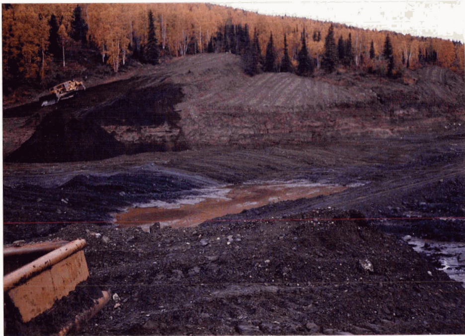
Active placer mining operation. Topsoil and overburden has been pushed to the valley side.
