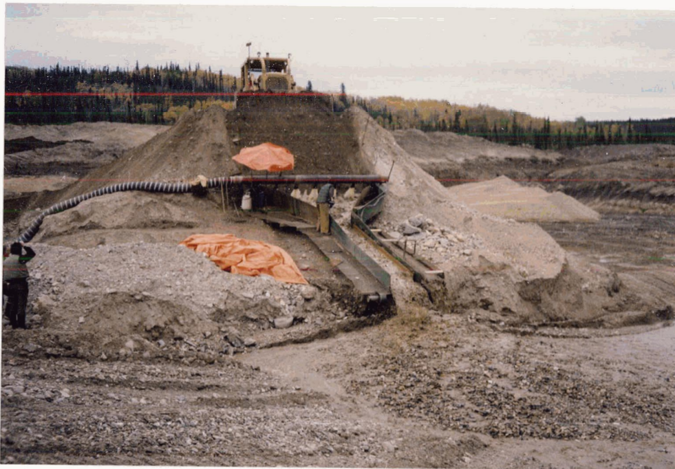
Sluicing operation. The fine soil particles are carried off with the process water, while the coarse particles are deposited at the base of the sluice box. Coarse tailings can be seen stockpiled behind the sluice.
