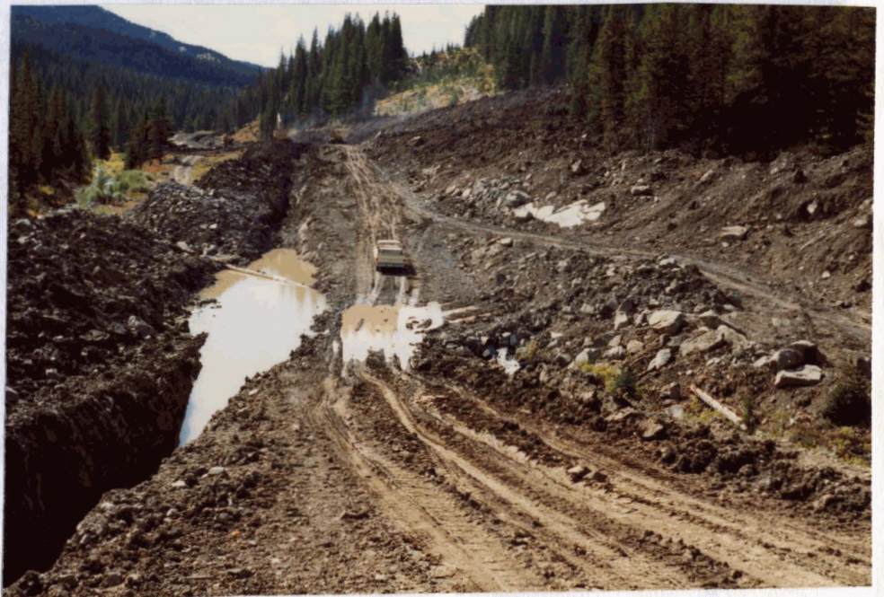
Figure 8: Right-of-way Drainage. Inadequate drainage on right-of-way while used as an access road. (Source: R.W. Langford)
