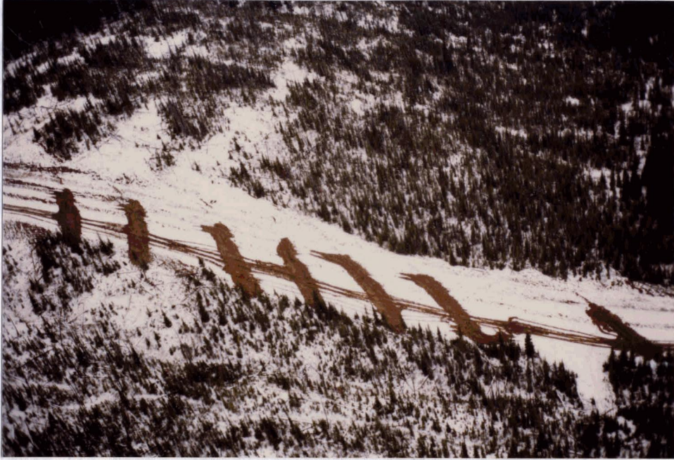
Figure 9: Berms Correctly Installed. Surface runoff is diverted from right-of-way into the trees. (Source: R.W. Langford)
