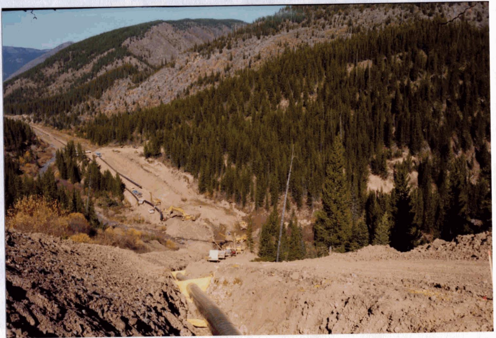
Figure 10: Ditch Plugs Correctly Installed. Plugs restrict water flow on steep slopes minimizing erosion of ditch. (Source: R.W. Langford)
