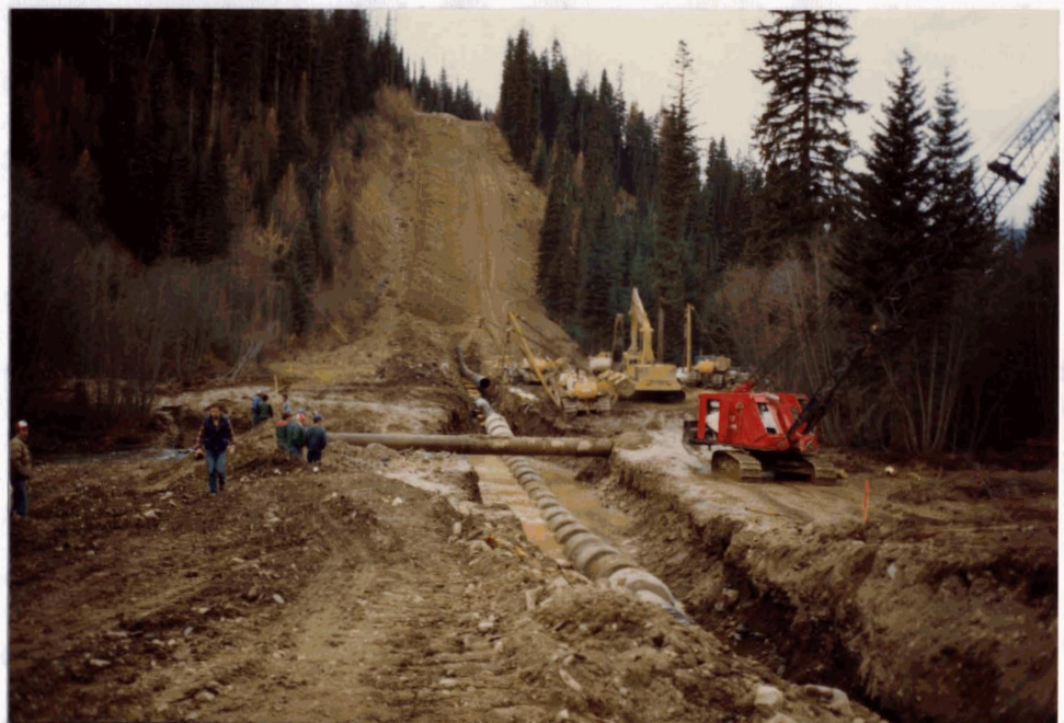
Figure 15a: Flumed Stream Crossing. Culvert carries all of stream flow across the right-of-way. Ditch is dug under the culvert and the pipe lowered in. (Source: R.W. Langford)
