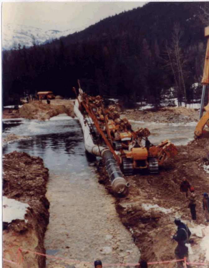
Figure 14: Open-cut Stream Crossing. Ditch has been excavated and pipe is positioned for lowering in. (Source: R.W. Langford)
