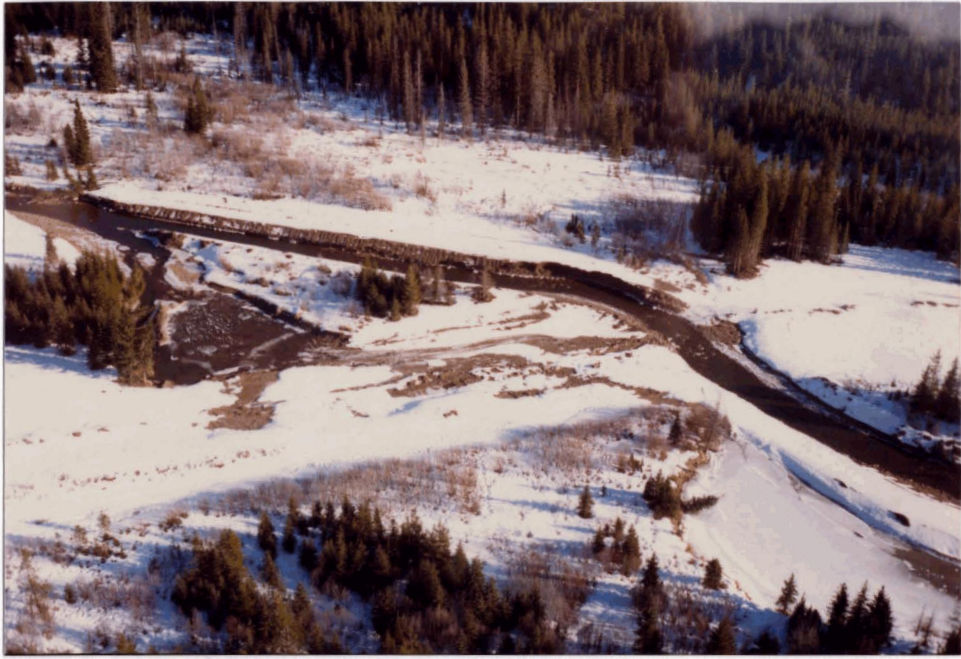
Figure 11: Inadequate Streambank Stabilization. Active cut bank in the centre of photo should be riprapped to protect right-of-way. (Source: R.W. Langford)
