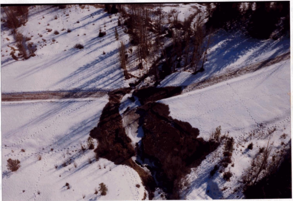
Figure 12: Inadequate Drainage on Access Road. Undersized culvert has washed out resulting in severe erosion. (Source: R.W. Langford)
