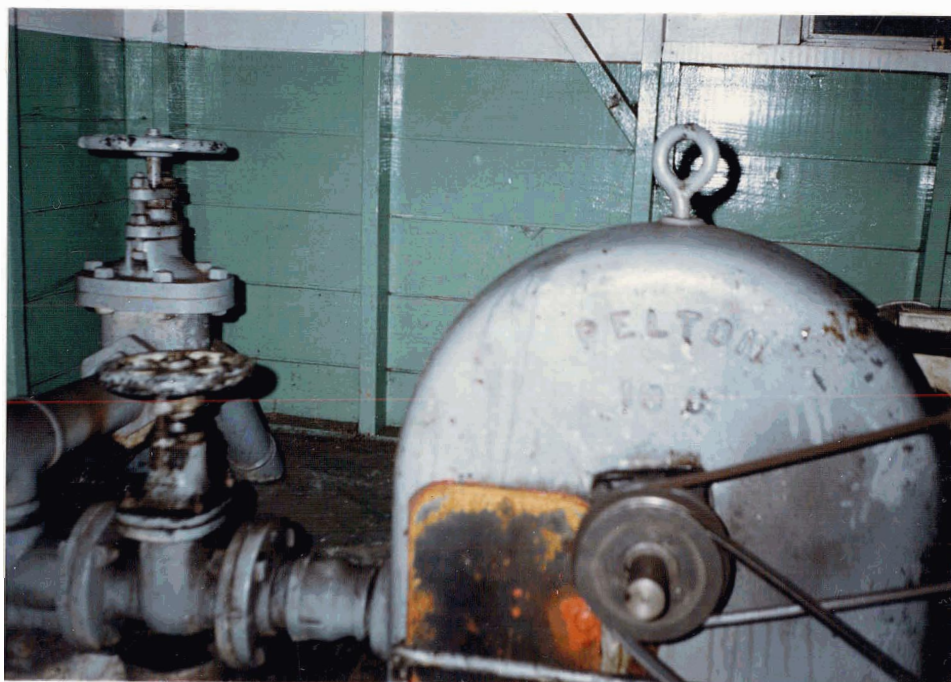
Plate 10: POWERHOUSE EQUIPMENT: Pelton Turbine Housing. (Koksilah Power Company, March 1986.)
