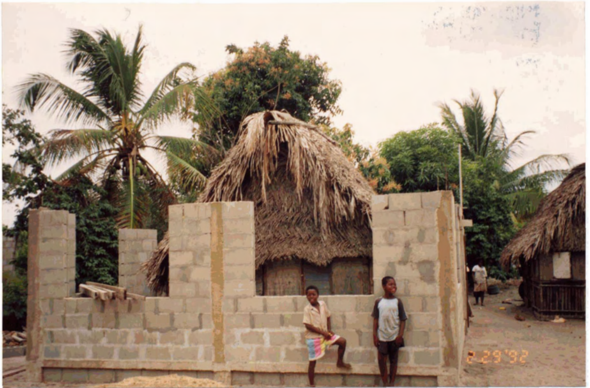
Figure 5.4: Concrete house being built around existing dwelling: two years into the job
