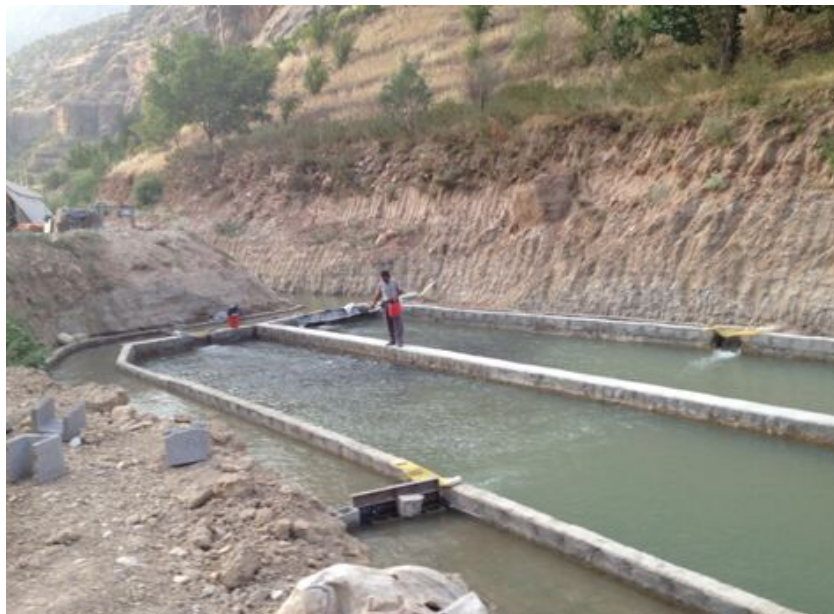
Figure 2.12. Unauthorized fish farm and orchard built on the side of the river in Sabzkouh (June 12, 2015). Note: This area is accessible by road. Community members alter lands with little fear of legal retribution.
