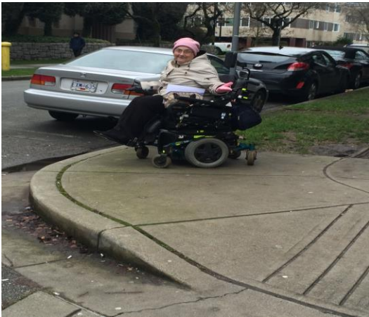
Incomplete curb cut
