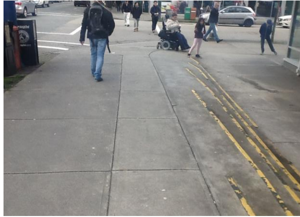
Dangerous sidewalk edging, Denman St
