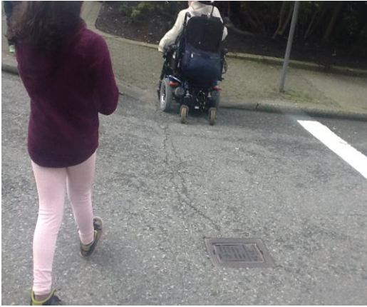
Uneven curb cut, Denman St
