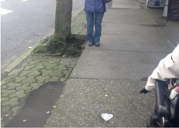
Exposed tree roots
