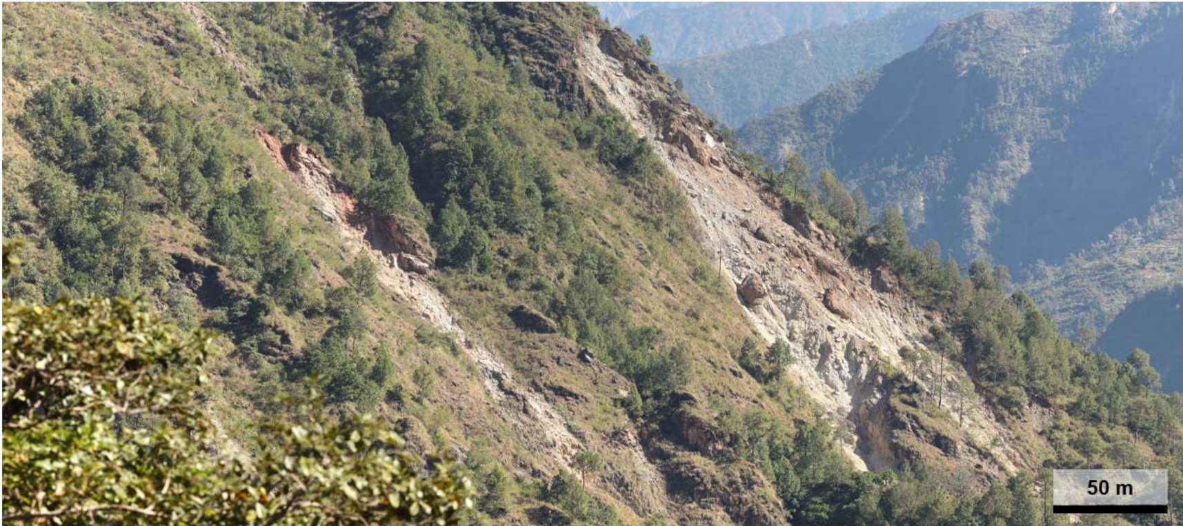
Figure H 8. Composite image of failures east of TLR as shown in Figure 5-2(e ,f) in main body of thesis. Created from photographs collected November 6, 2016 looking north-east.
