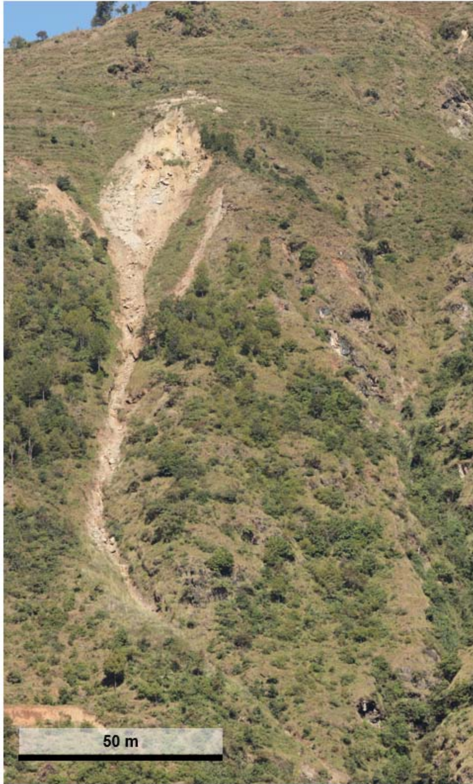
Figure H 5. Composite image of failure west of TLR as shown in Figure 5-2(b) in main body of thesis. Created from photographs collected November 6, 2016 looking north-west.
