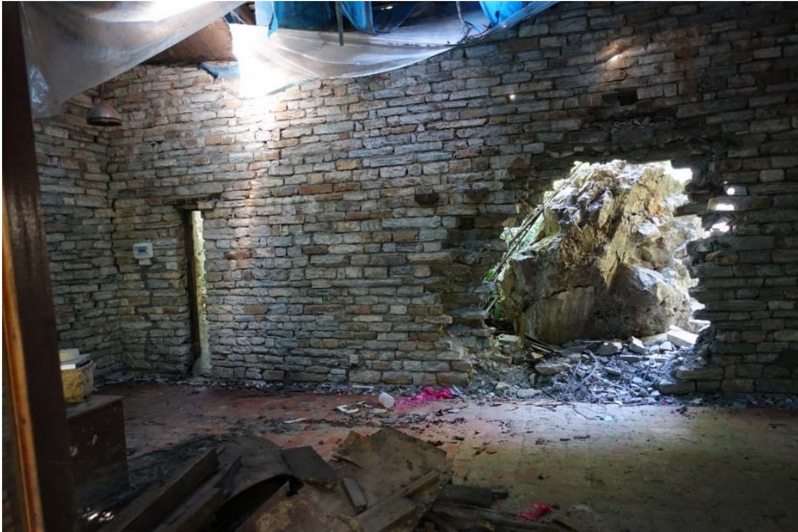
Figure H 1. Brecciated boulder lodged into the back of the spa facility at TLR. Boulder is approximately 2 m tall and 3 m in length. Photograph taken November 13, 2016.
