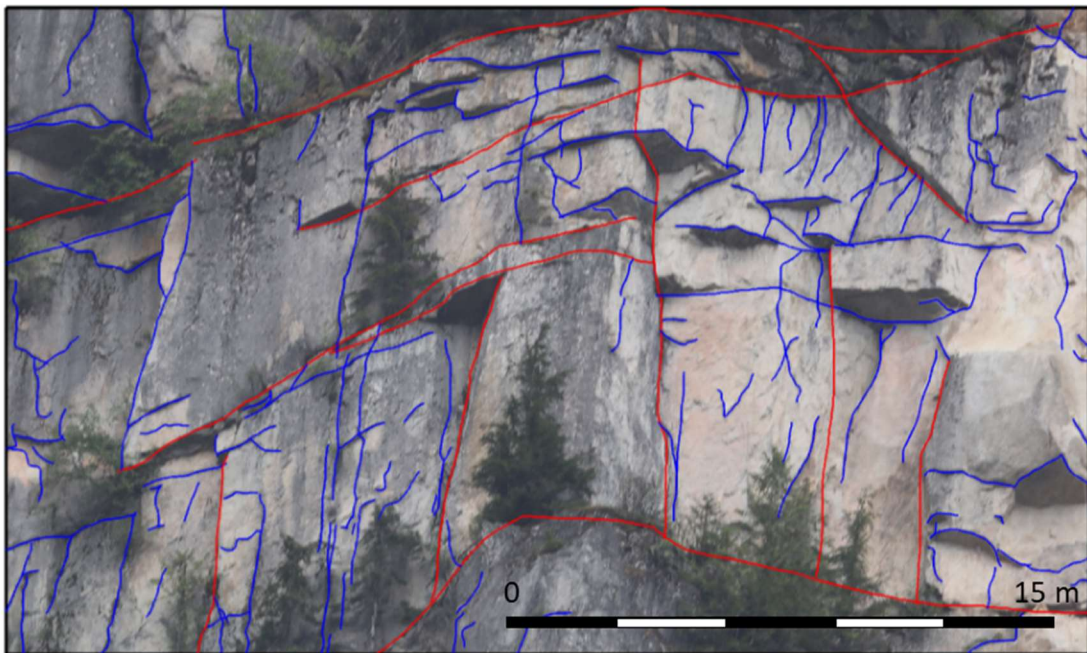
Figure A5: Chief damage mapping window 4
