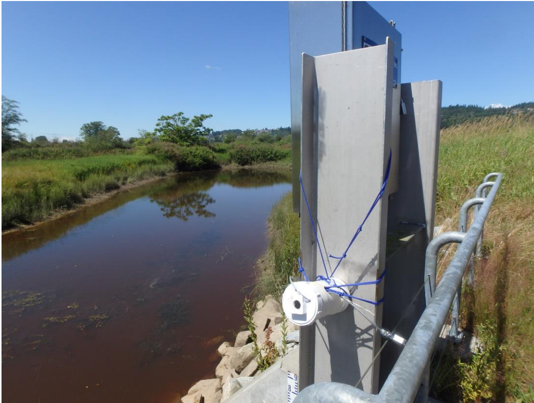
Figure A3. An example of camera installation: Here the camera was locked to a railing above the floodgate. Ropes were used to angle the camera into a good position to focus on the floodgate below. At other sites, pieces of foam and zip ties were used to adjust camera angles.
