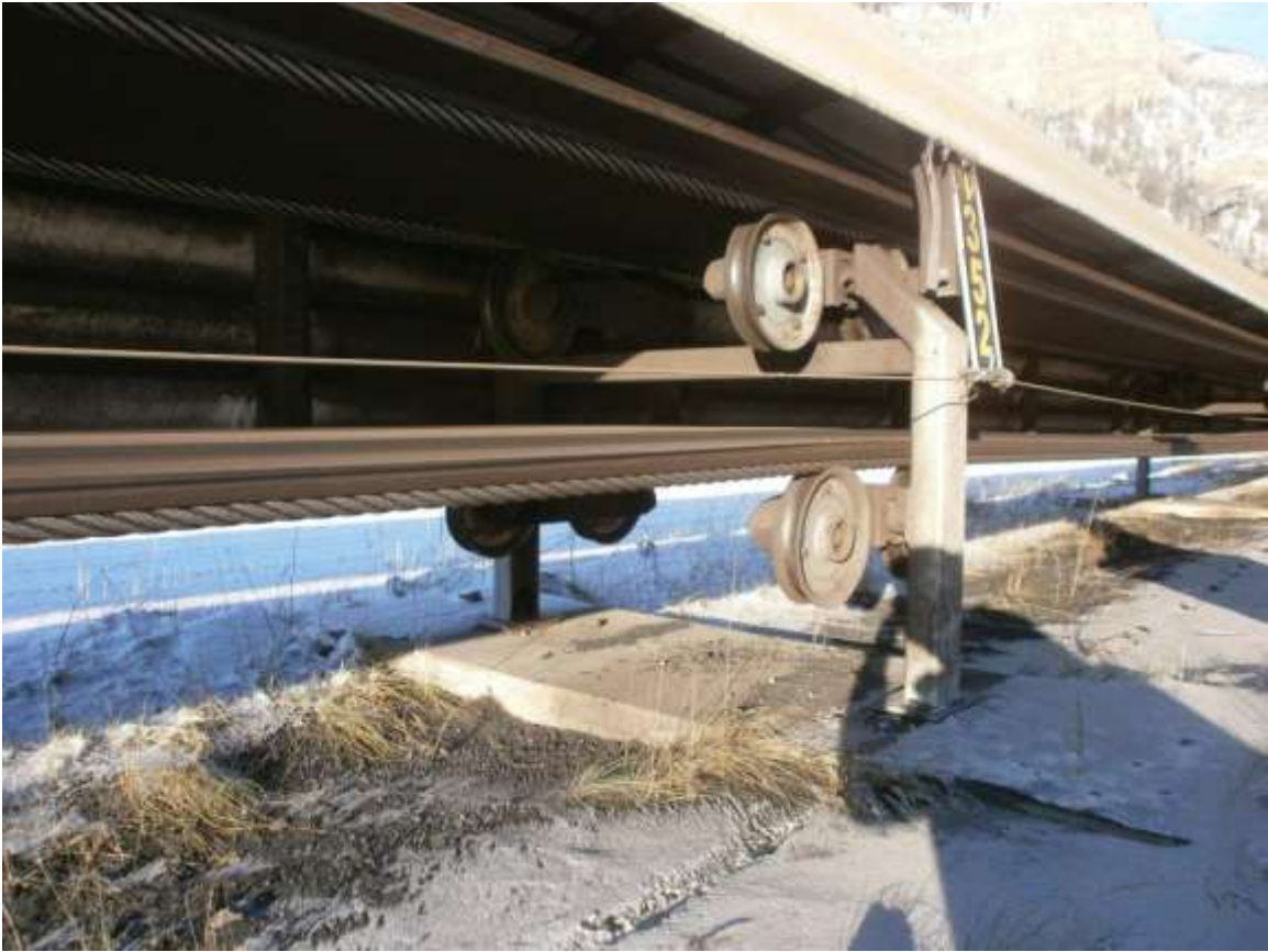
Figure 4-1 Line Creek Operations Cable Belt
