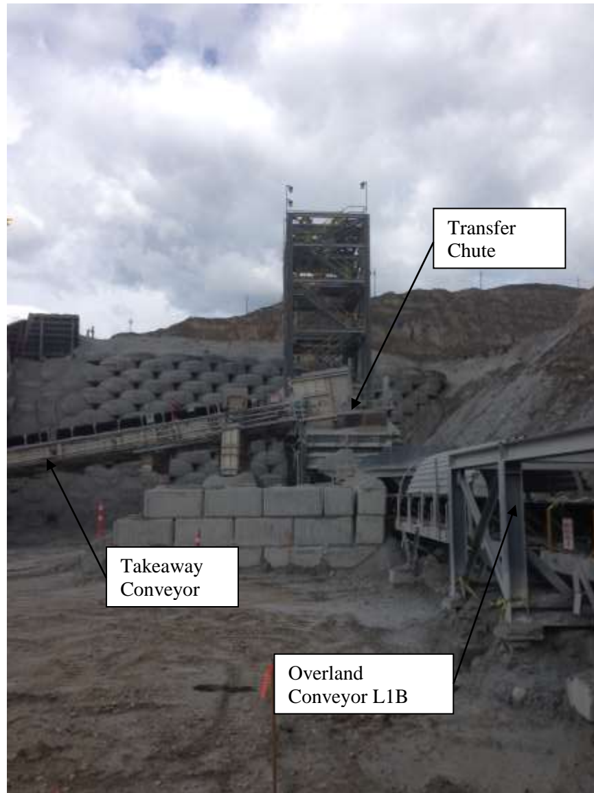
Figure 4 Transfer Station onto L1B Conveyor (by Author)
