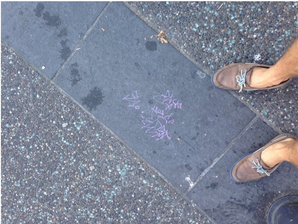
Figure 18: Granville Street granite paving vandalism (Source: L. Hoyt, 2013)
