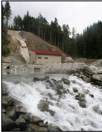
Figure 8. Fitzsimmons Creek IPP Powerhouse and Snowmaking Intake Pond (Ecosign Mountain Resort Planners Ltd., 2010)
