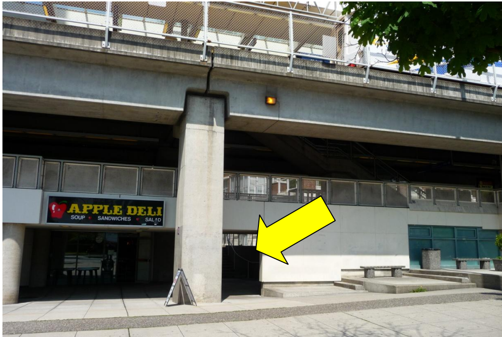
Figure 22 – Access between Station entrance and City Gate, south side, May 31 2011 (Source: © A. Jones)
