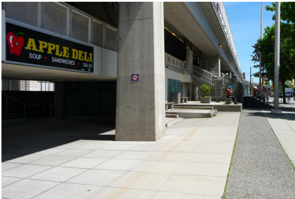
Figure 23 – Access between Station entrance and City Gate, south side, June 4 2011 (Source: © A. Jones)
