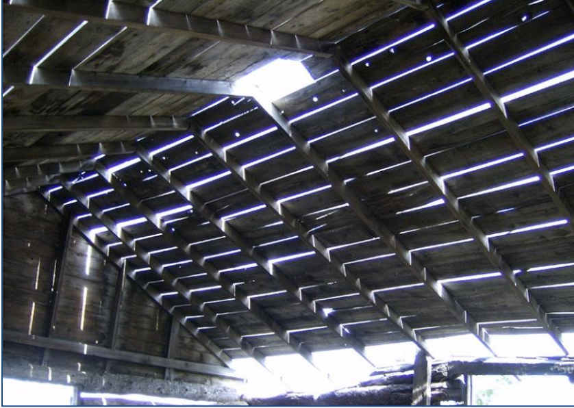
Figure 33. Inside the One-Owl cabin, looking at the chimney hole. Photo by author.
