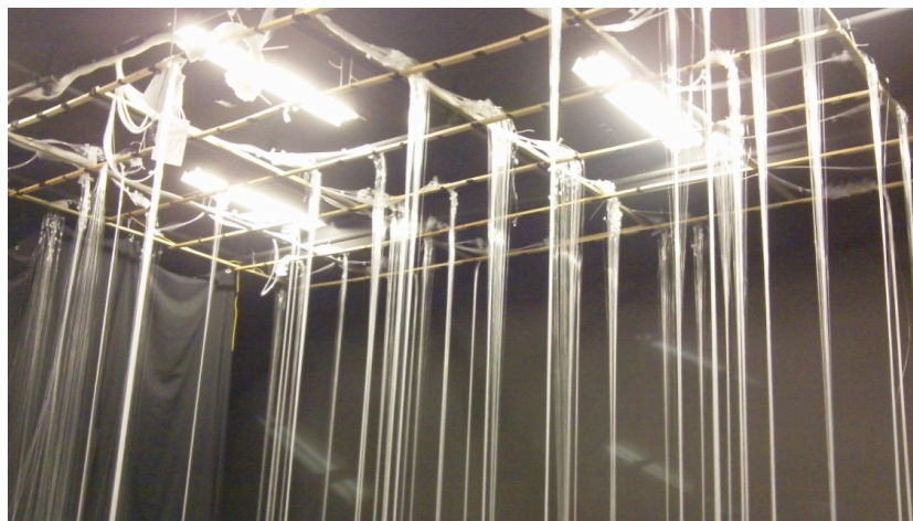
Figure 41. Ceiling grid for hanging fiber optics
