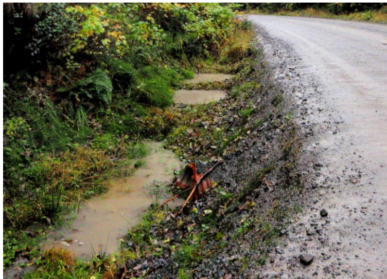
Figure 4.4 Sediment laden road surface runoff passing through ditch blocks along the Queen Charlotte Mainline Forest Road South
