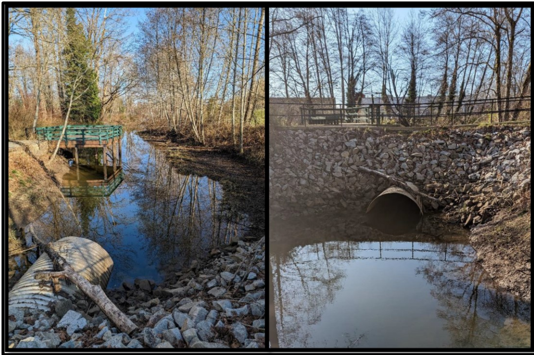
Figure 5: Simms Creek study site. One of the pool features (left), and the new “fish friendly” culvert as seen at high tide when fish can pass in between the pools and the Courtenay River (right).
