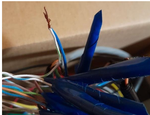
Figure 2.8: Suspected Cause of Unstable Connections and Sensitivity Issues
