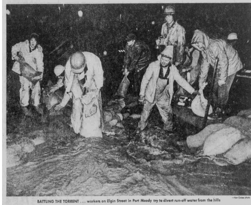
BATTLING THE TORRENT . . . workers on Elgin Street in Port Moody try to divert run-off water from the hills —Ken Oakes photo
