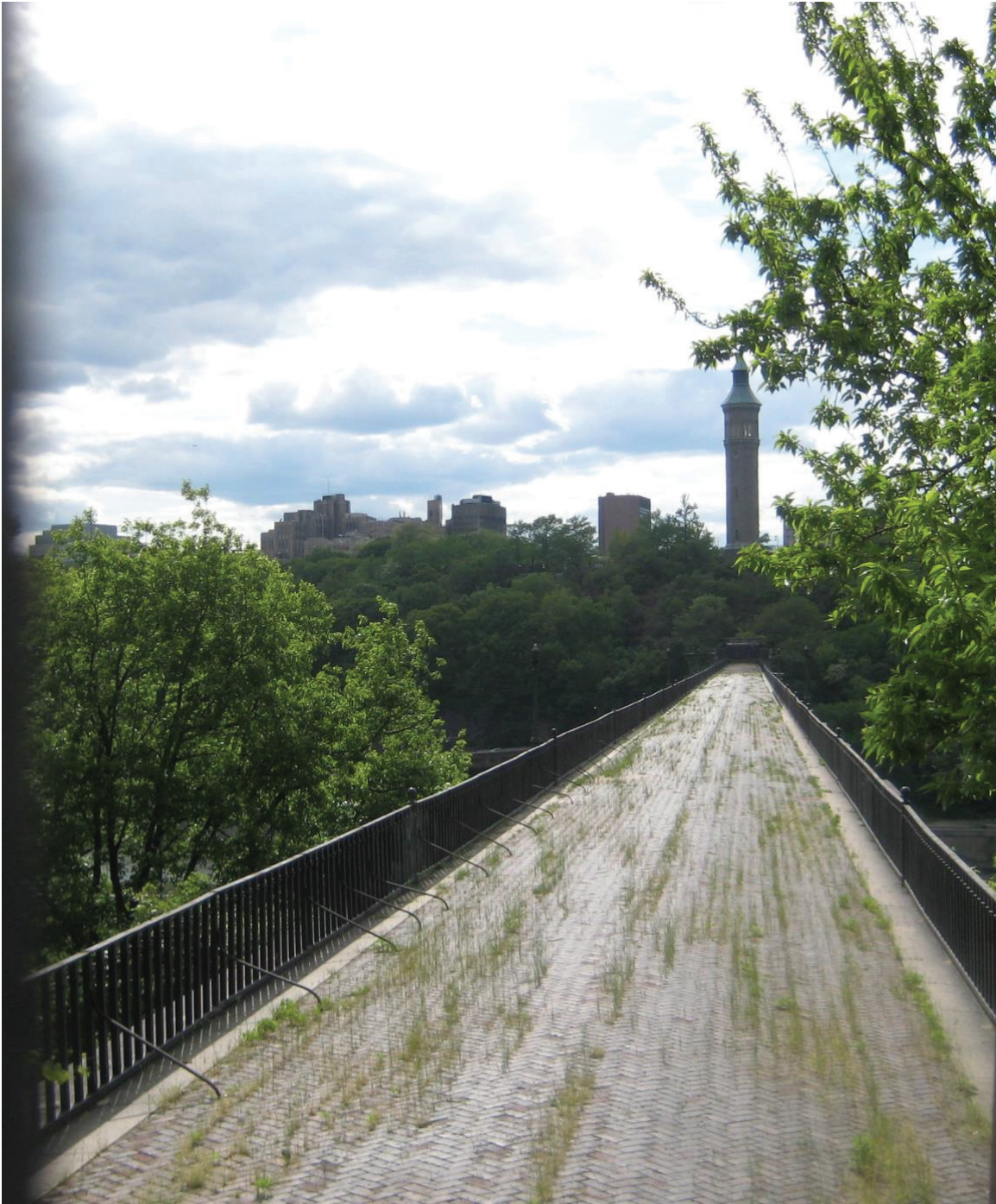
Figure 1.1 View West from Highbridge, Bronx to Manhattan over the High Bridge prior to restoration.
