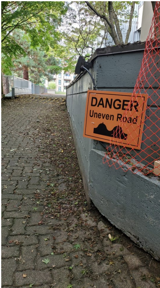
Figure 5.5. Fountain Way uneven road
