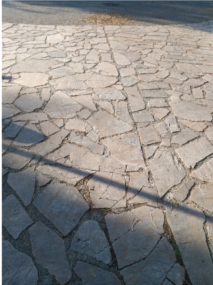
Figure 5.3. Flagstone pavers: Fall hazard
