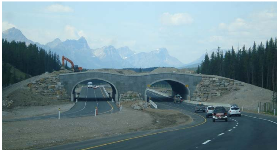
Figure 8. BNP Animal Crossing: Photo showing one of the new wildlife corridor overpasses under construction in August 2009. (Source: Billy Collins)
