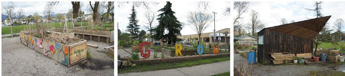
Figure 7.4. Le Chou bed (left), garden fence (middle), and the tool shed (right) built by CityStudio students.
